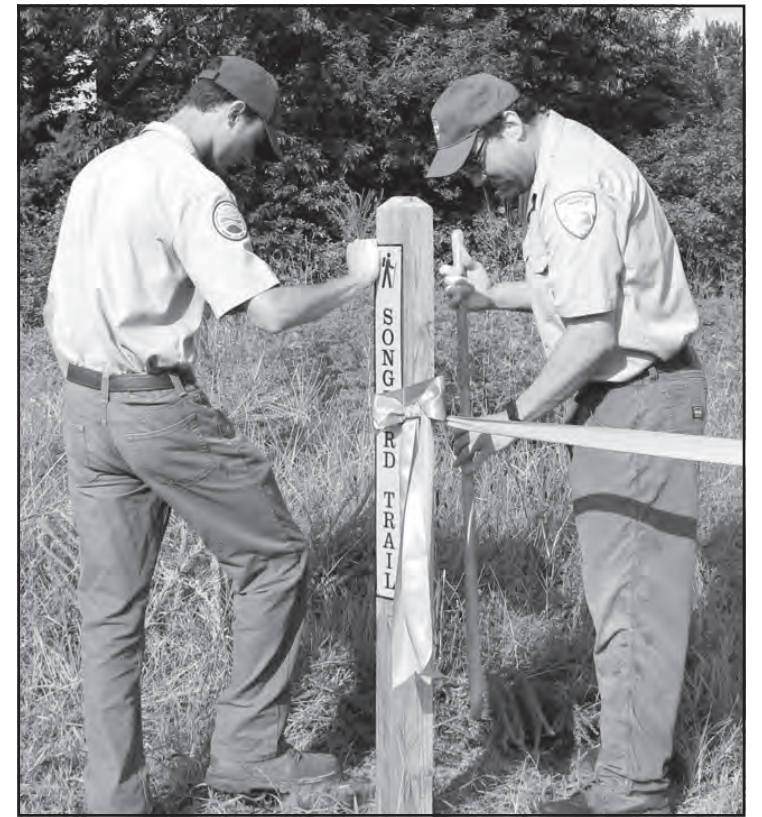
C.J. Bailey and Shaun Vest finish the installation of the post at Machicomoco State Park's Songbird Trail.
