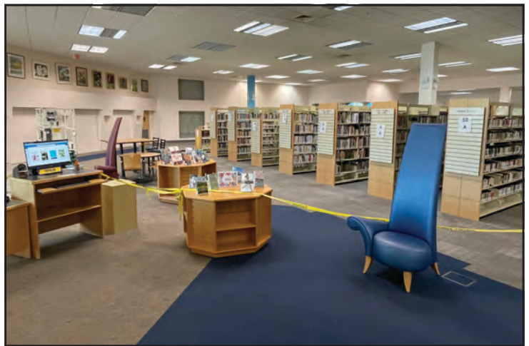
Renovations are underway at Gloucester Public Library, Main Street Center branch. Work is expected to be completed by the end of May.
